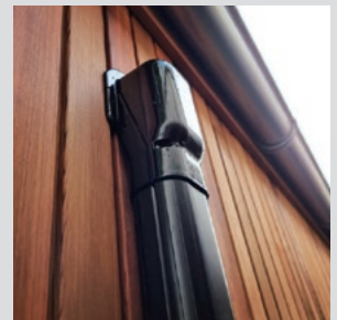
Photo provided by JMG Cooling Services (UK)
