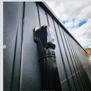
Photo provided by JMG Cooling Services (UK)
